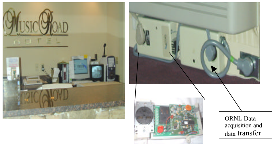
Fig. 5. Clockwise from left: front desk controller at motel, installed Digi-Log unit and controlboard, ORNL data processing and data transfer module.
