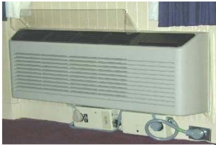
Figure 4.3 The Digi-Log PTAC controller (box below the PTAC and on right) adds central control capability to existing hotel/motel heating and cooling systems. An ORNL data collection box is located to the left.
