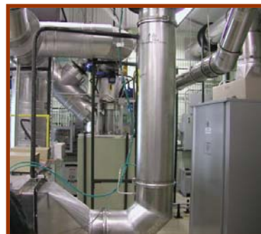
Absorption Chiller (On Right)
