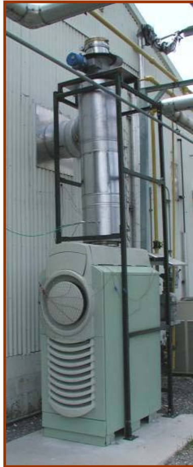
Figure 10.2. A 30-kW Natural Gas-Fired Microturbine (Located Outdoors)
